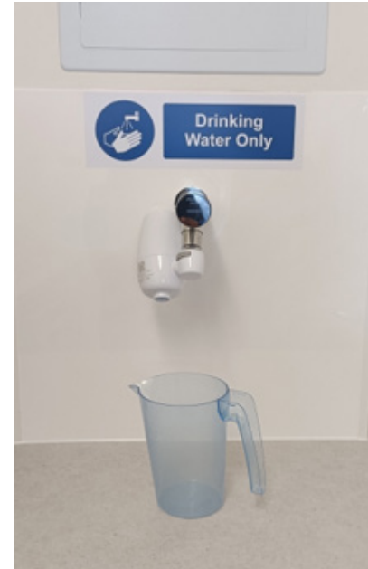
After: "Drainless" outlet (Frimley faucet)
